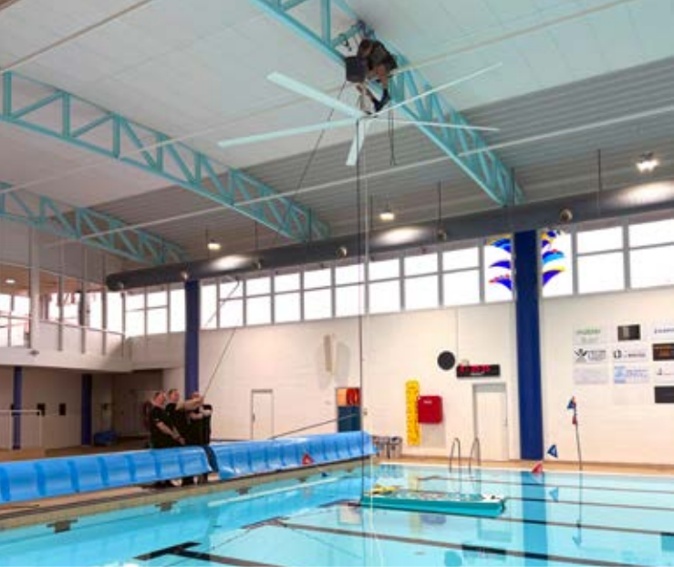
February 2023, where 2 large HVLS fans from Nordicco are being installed by a professional climbing team.
