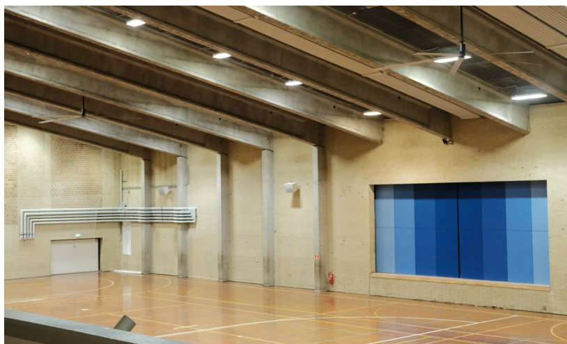
Høng Sports Facility with two NORDICCO fans installed.
