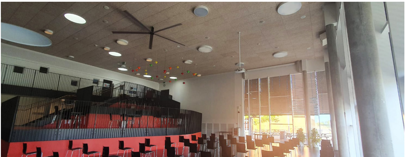
The fan helps to ensure an improved indoor climate, benefitting both students and employees at the Høng School.
